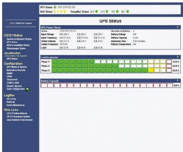
Configuration and monitoring via web browser
